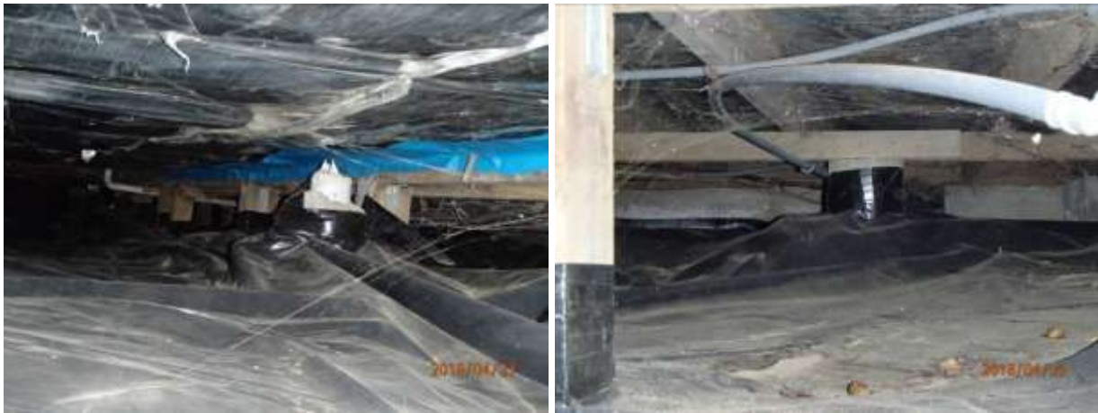
Polythene over the ground is dry, butylene plumbing, pvc wastes, all good
