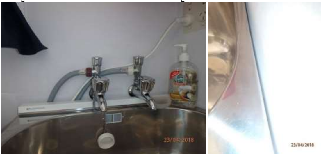
The tub is not secured or sealed to the side wall.
