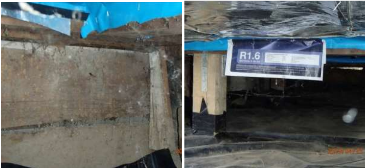
Borer damage in base boards behind plaster. R1.6 insulation
