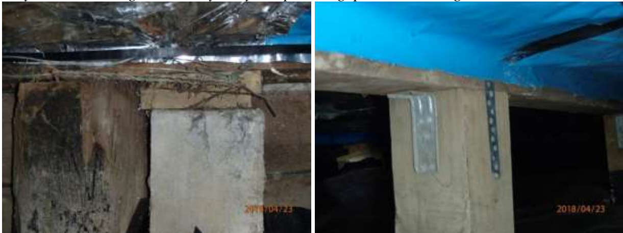
Old Totara pile, old concrete pile and now all new treated timber piles with great fixings.
